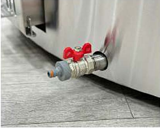
Water outlet from side
